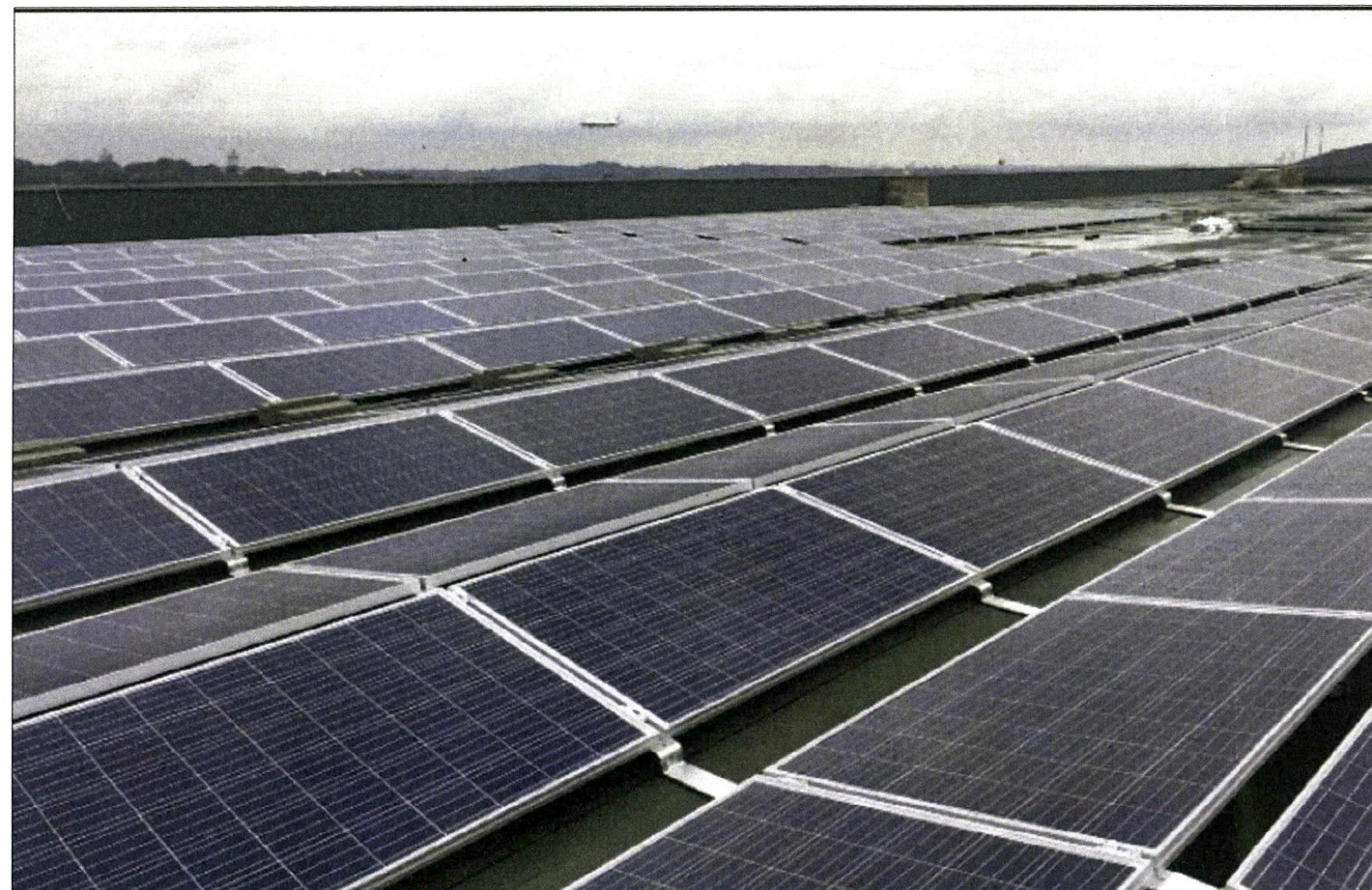
Image of typical PV array (East & West facing)
